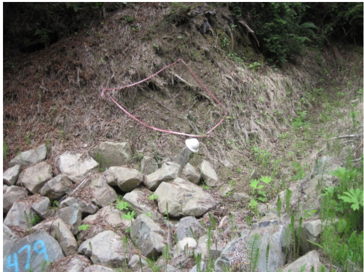
Figure 4. Erosion void measurement of bank slough
