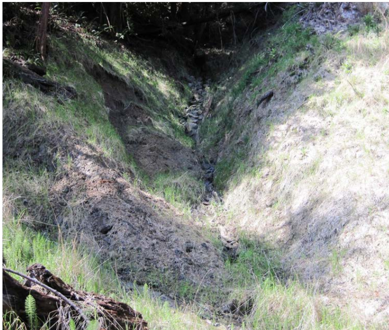
Figure 32. Slope failure adjacent to newly excavated channel.
